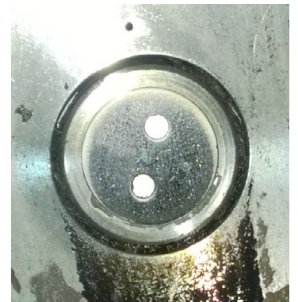
Sensor after one year of operation shows no scaling on sensor surfaces
