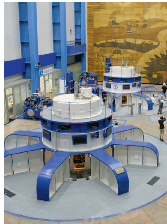
Unit #1 and unit #2 after modernization
